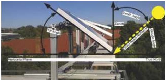
Figure 5: Different tilt angles visible on this PV array where one singular Zenith Angle exists
