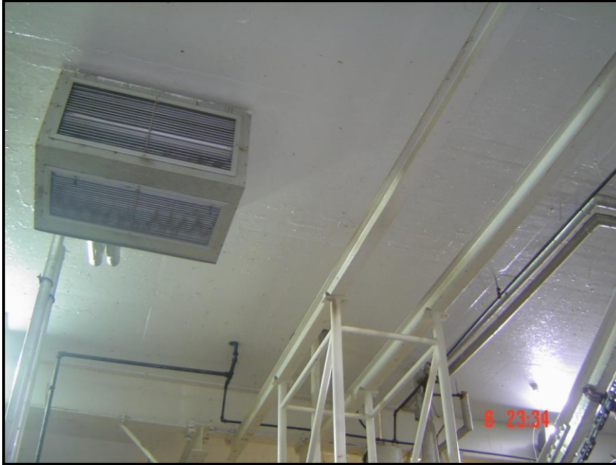
Figure 2.14: Air conditioning device situated below the ceiling
