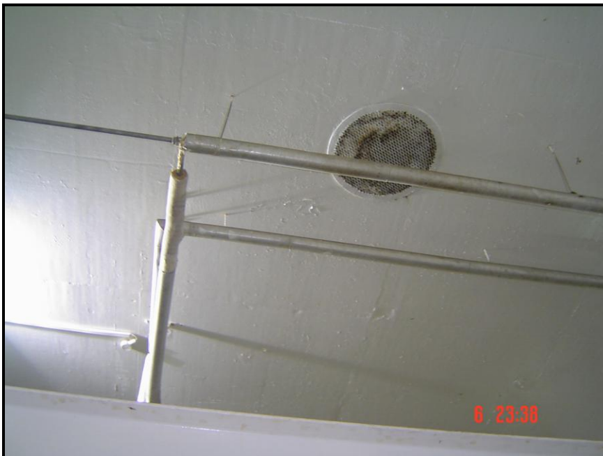
Figure 2.15: Extractor fan situated in the ceiling
