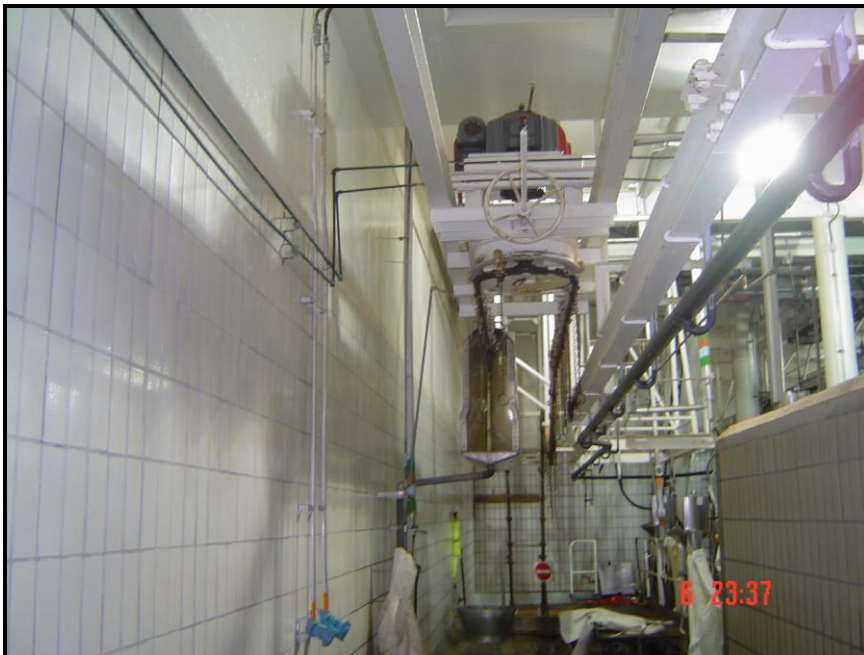
Figure 2.13: Motor used to operate the conveyors
