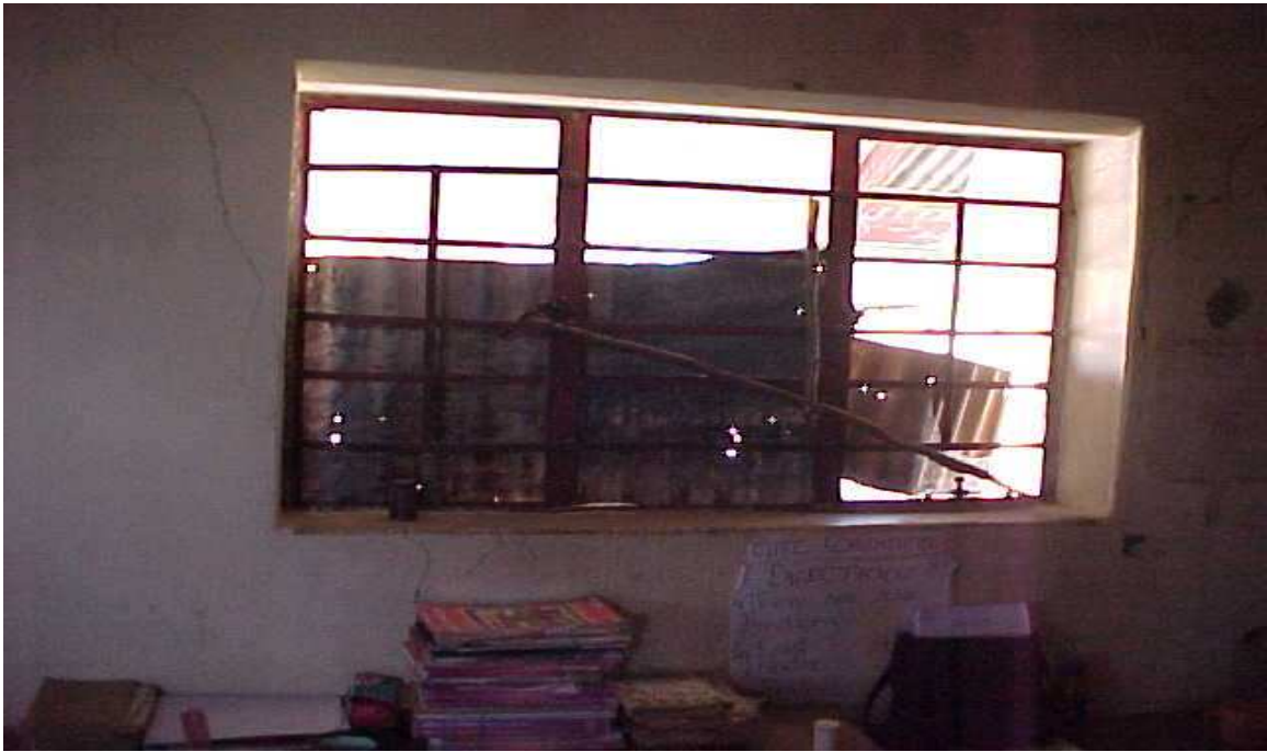
Figure 1.5 Broken window in a primary school taking part in the primary school feeding programme
