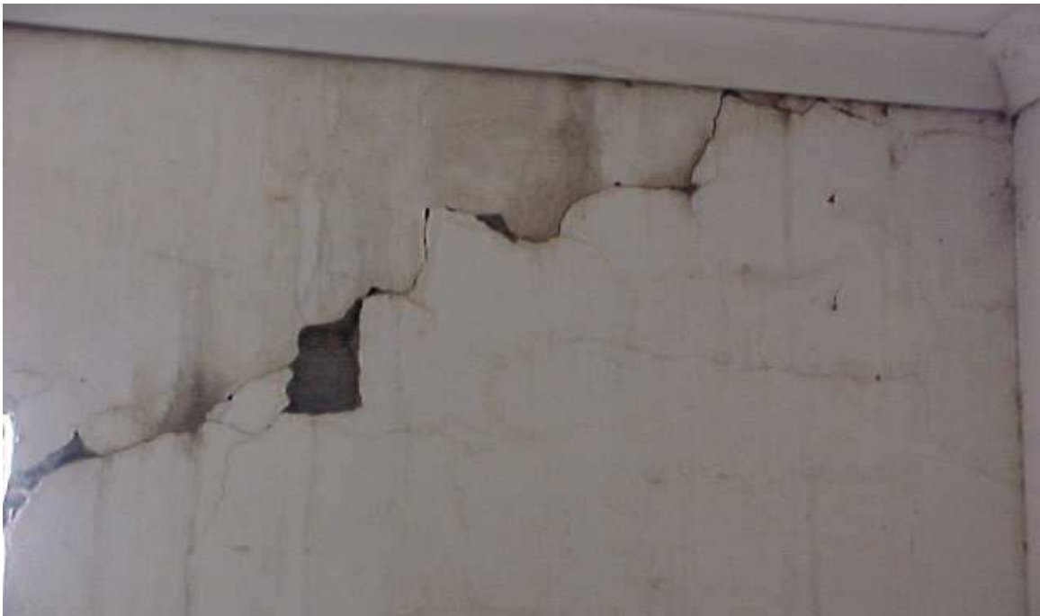
Figure 1.6 Cracked and moisture-damaged wall in a storage room of a primary school partaking in a feeding programme
