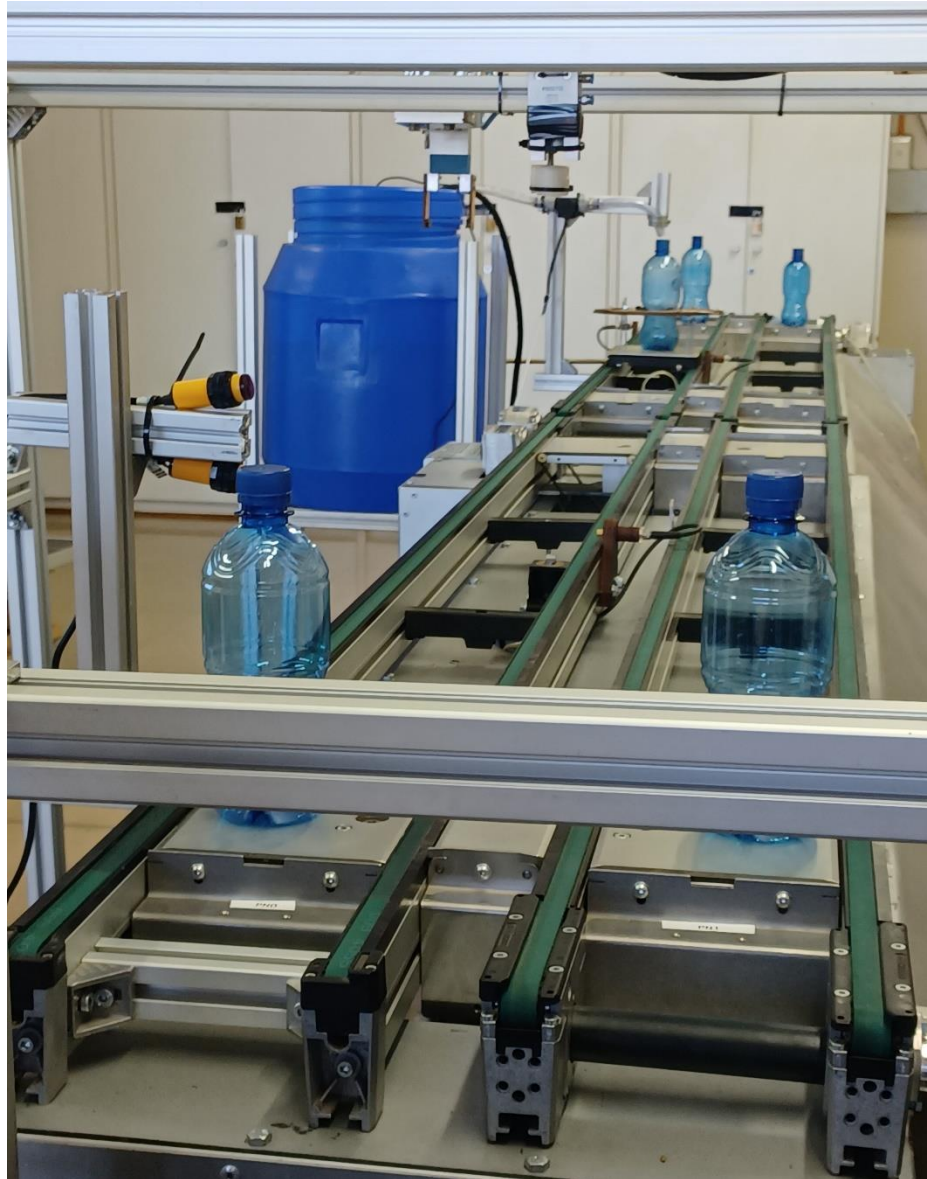
Figure E.1. The water bottling plant in operation.
