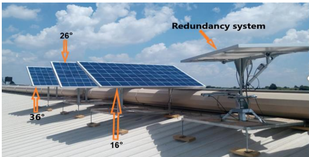
Figure 4.5. The three fixed PV modules.
