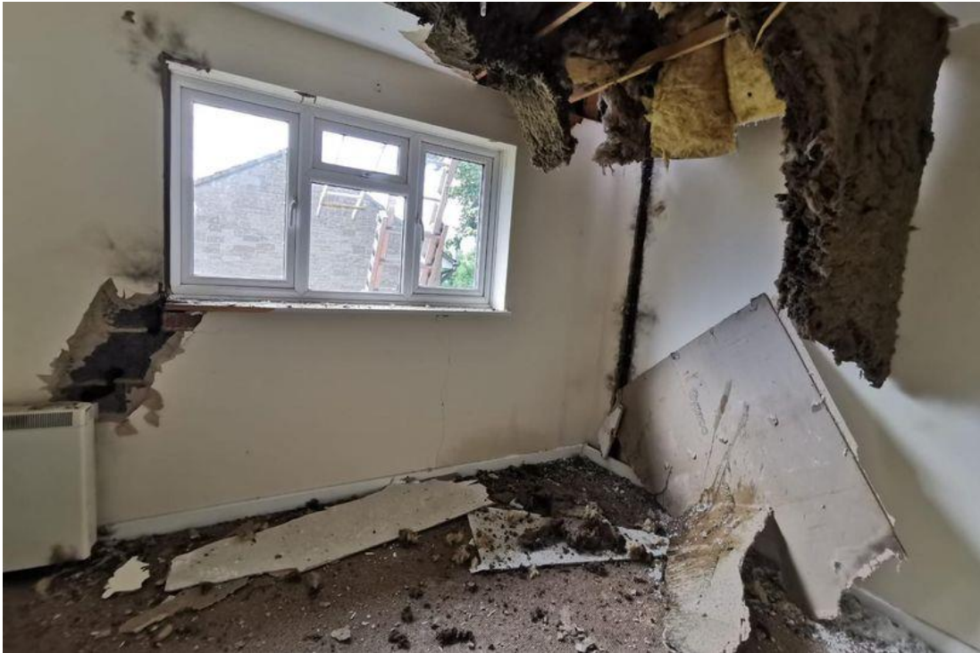
Figure 5: Direct lightning strike damage to house [27]
