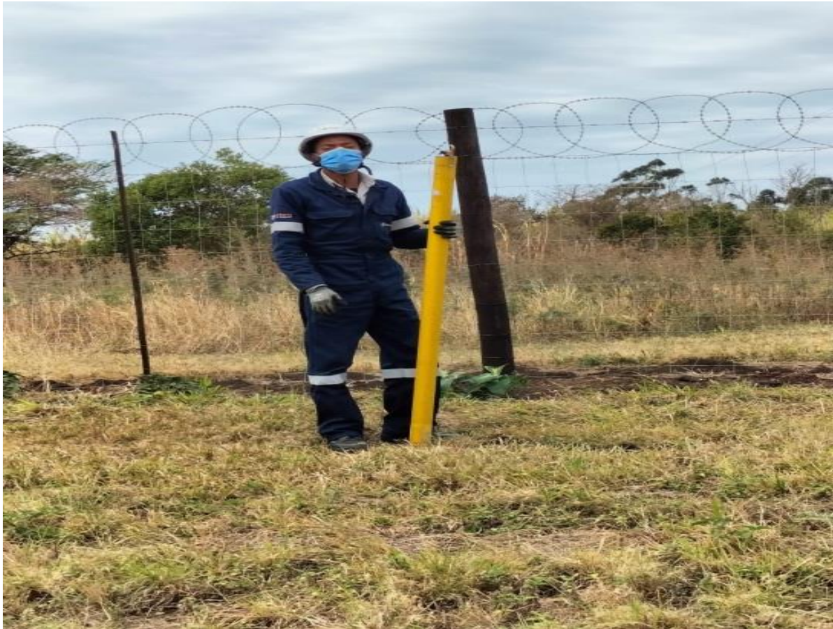
Figure 17: Suitable condition of ppe worn by workers before replacing a fuse
