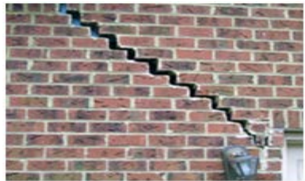
Figure 6. Crack at the corner of the wall opening due to foundation differential settlement caused by heaving soils at Winburg
