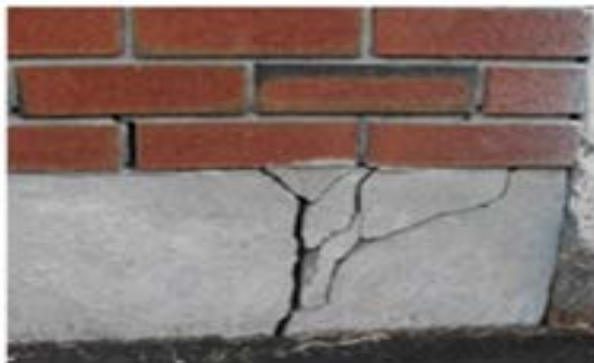
Figure 5. Buckled foundation defect from heaving soils at Kroonstad
