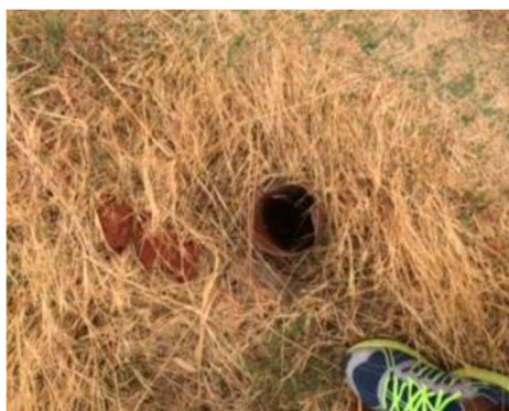
Figure 10. Poorly constructed borehole in the southern landfill site.
