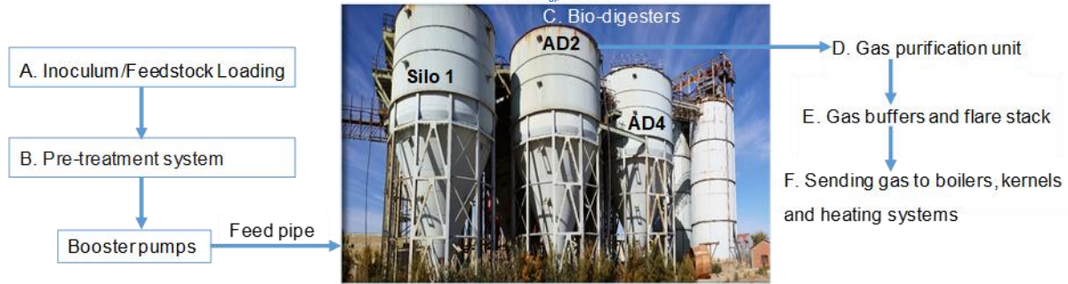
Figure 5: Visual representation of the process flow of the bio-energy plant. The feed/inoculum was delivered into the pre-treatment system (A), where it was mechanically treated (B). The booster pumps were responsible for pumping the feed/inoculum via a feed pipe into the digester (AD2, with a volume of 1200 m 3 ) (C). When gas was produced, it was directed to the gas buffer tanks after purification (D). Two buffer tanks ( \approx 10\,000\text{ m}^3 each) were used to store the gas.
