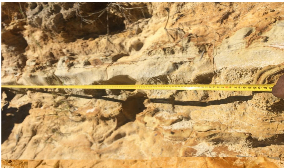
Figure 6.3: The side view surface of the dam with cracks and fissures.
