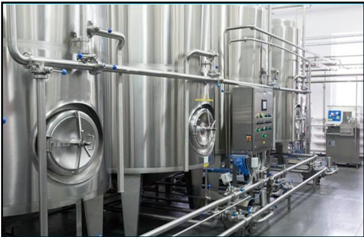
Figure 2.2: An example of a CIP system with all connecting pipelines for dosing, mixing and circulation of disinfectants during disinfection with the required valves, spray balls, hatches and PLC screens for monitoring and control
