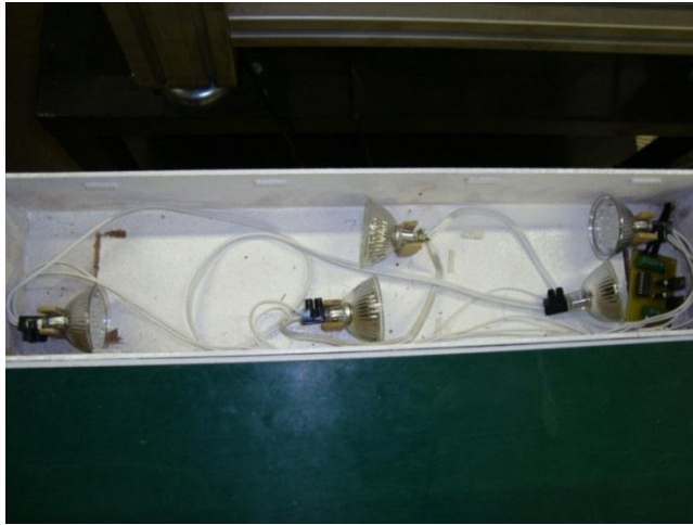
Figure 5.9 Inspection bay with 50 W halogen lamps as a light source
