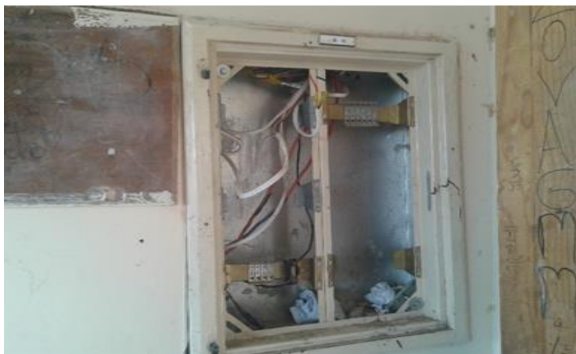
Picture 5.10: Circuit breakers removed from the main switch at school C
