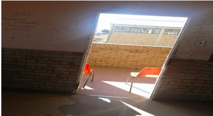
Picture 5.12: A classroom without a door at school F
