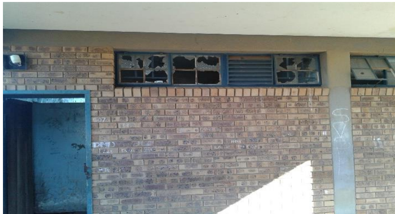
Picture 5.4: Broken toilets windows at school E
