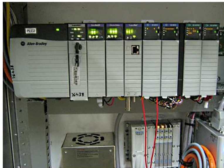
Figure 2.2: Allen-Bradley Module Backplane
