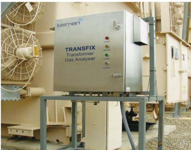
Figure 4: A gas analyzers installed in transformer [11]
