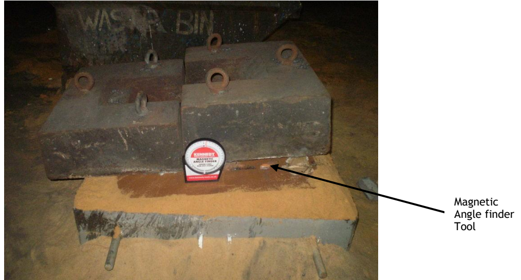
Figure 5: Assembled mould with weights and required inclination (see magnetic angle finder tool) ready to be poured.
