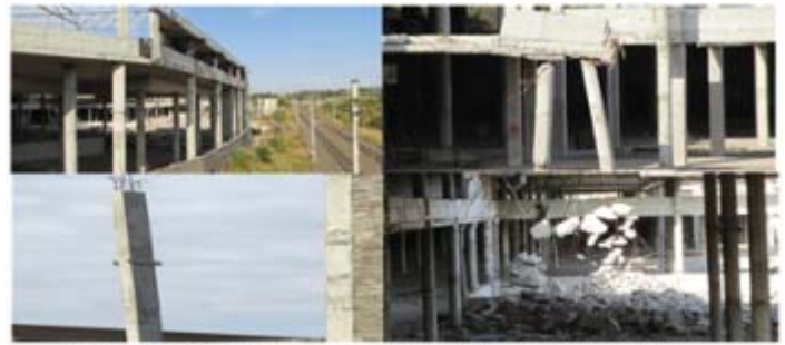
Figure 6: Recorded cracks and deflections in the collapsed building
