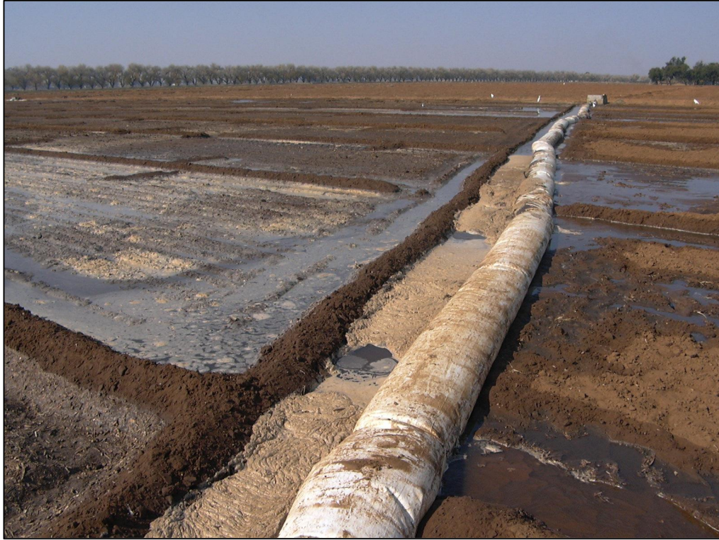
Picture A3: Flood irrigation from community canal 5 F.
