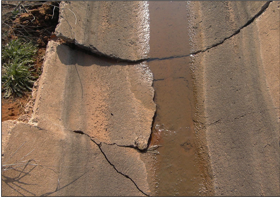
Picture A7: Water losses due to seepage in community canal 5G.
